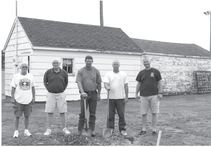
From left: Al Siems, Duane Nevenhoven, Nolan Junker, Brad Eiklenborg and Brent Siems stand in front of the concessions stand at the Stout Astrodome. The installation of a water main marks the beginning of the process to replace the former brooder house with a brand new concession stand and bathroom facility. (Greg Forbes/Mid-America Publishing Photo)
